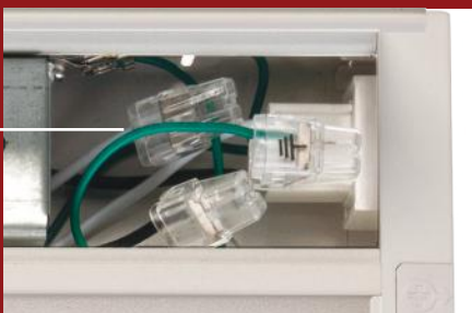
Ample Wiring Space
